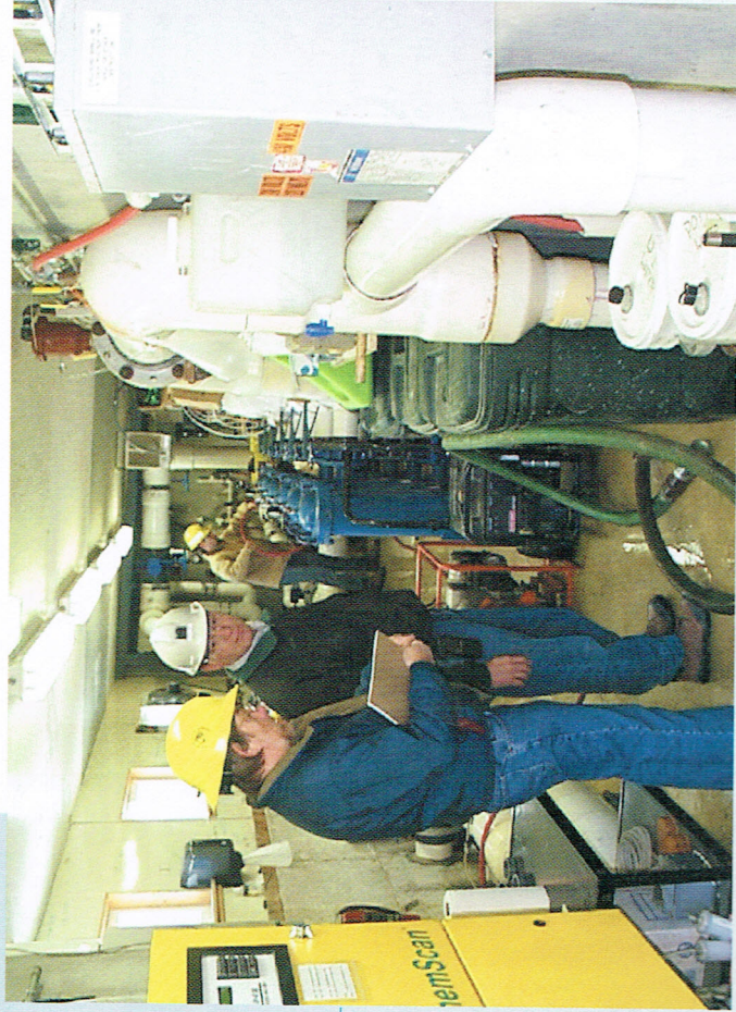
The Anoxic Biotreatment Cell (ABC) process support building houses pumps, flowmeters, filters, valving, an on-line nitrogen analyzer and other controls.
