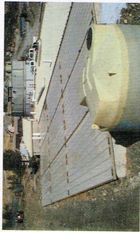
The full-scale Anoxic Biotreatment Cell (ABC) consistently has removed over 90 percent of the incoming nitrate and has a treatment capacity of 1100 gpm.
